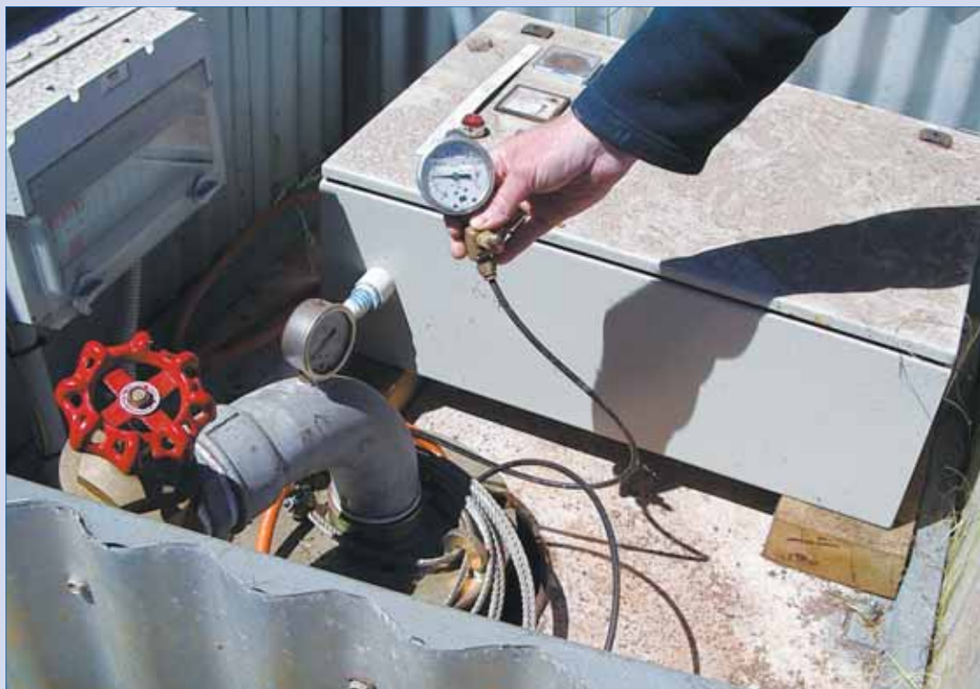
A simple water level gauge will cost around $150, but could save tens of thousands.
