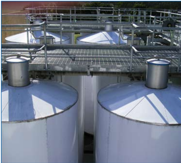
Pipers Brook's outdoor storage tank farm
