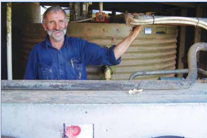
Duncan Sadler with his ice bank in the background and compressor in the foreground.
