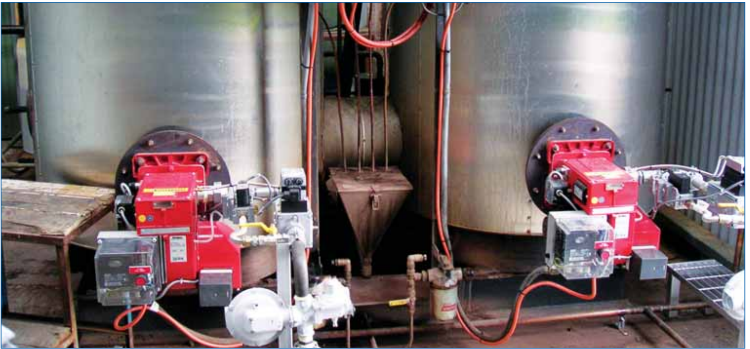
Gas fuelled boilers.
