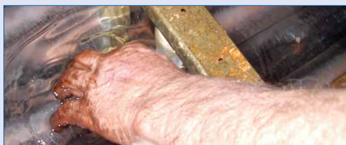
Inside an ice bank - showing ice forming along the outside of the evaporator coils.
