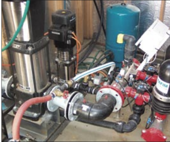
Pumps to operate the polyhouse and the outdoor irrigation systems.
