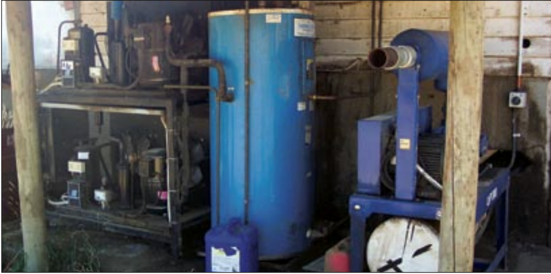
The Therma Heat Recovery System.
