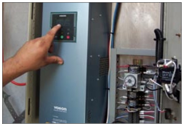
Vagon variable-speed drive-control box.
